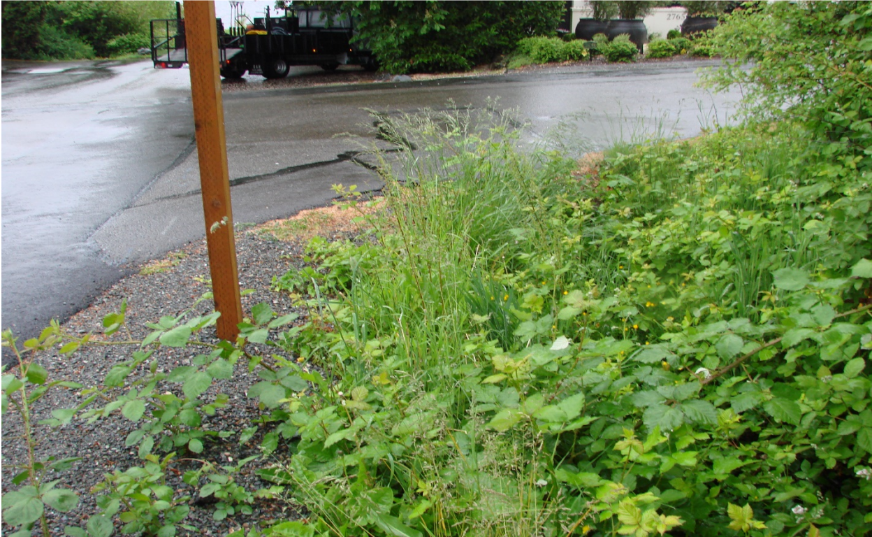
Photo #9 – Open ditch inlet at northeast corner of SE 28 th Street & 60 th Avenue SE
