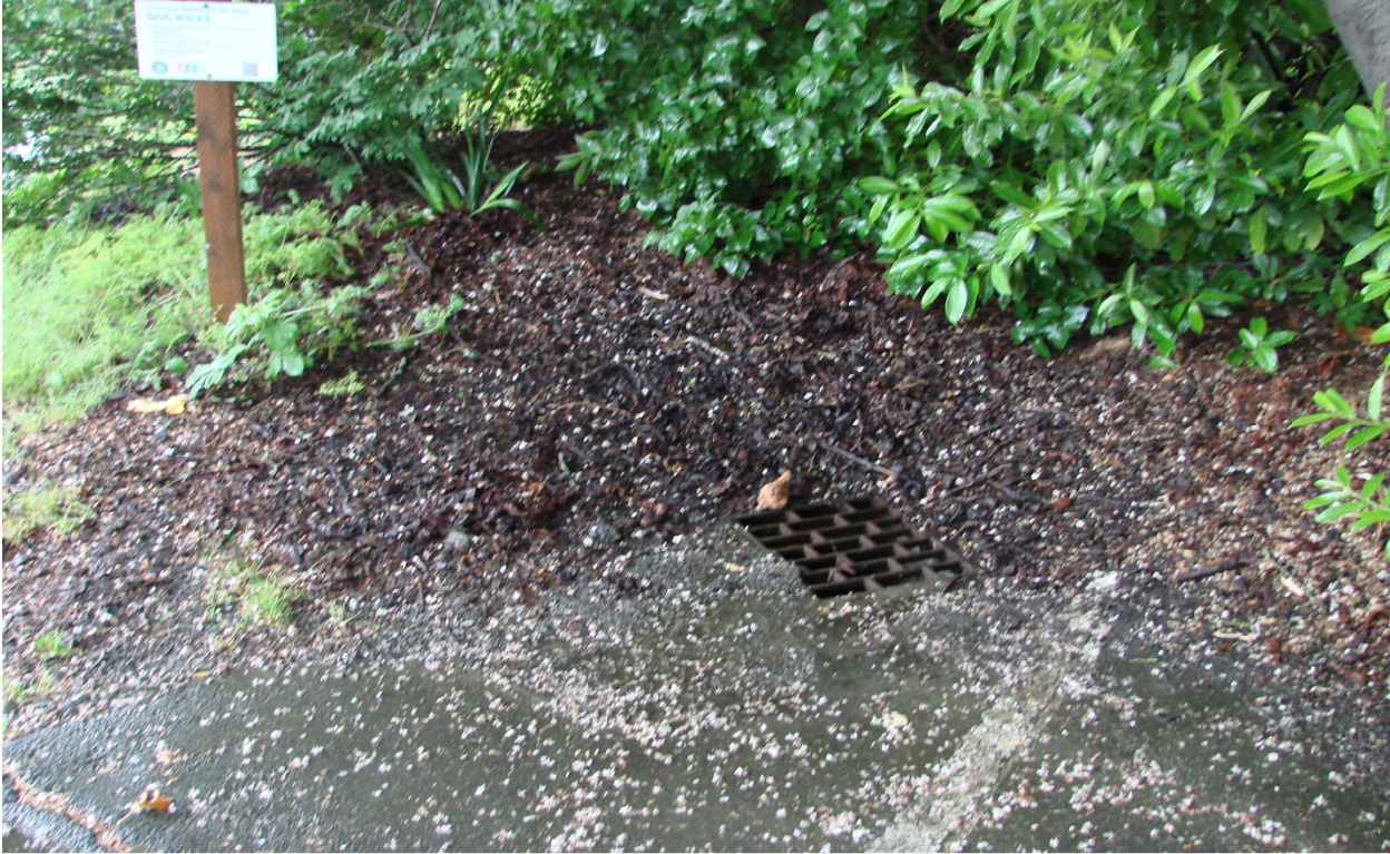
Photo #10 – City CB #16-11 within parking area of Calkins Landing Park (north side)
